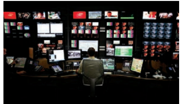
Custom Consoles' Media Wall display is action at the Associated Press TV facilities in North London, UK
