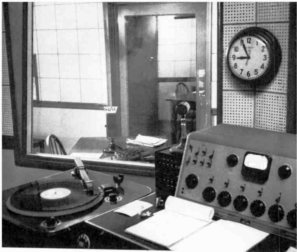
An early control room with record turntable and console.
