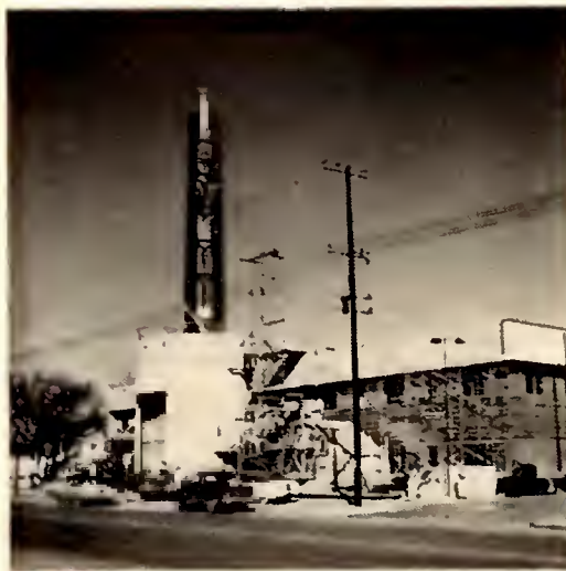
KVOO & KVOO-TV, Tulsa, progress picture of new broadcasting plant. Unique tower will stand 172½ ft. when completed, serving as microwave receiver for remotes.
