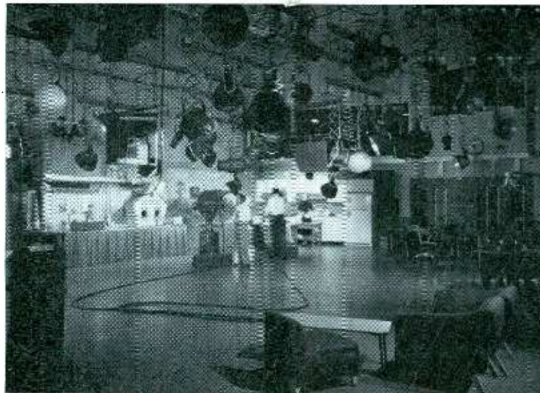
Noteworthy is the design of the two large WSB-TV studios. An interesting aspect of construction is the square power ducts, running the lengths of the studios and suspended by bolted bars from the joists. Electrical cables feed boom-like pipe supports which in turn hold pantographs with the many kinds of spotlights required for TV. Roof deck is Tectum, providing sound absorption.
