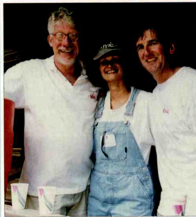
For Time magazine's recent day of community service, staffers turned out to renovate Camp Minisink in Dover Plains, N.Y., serving children from Harlem and the South Bronx. (L. to r.) Jim Quinn and Maria Orenge, of NYC Mission Society, the camp's founding organization; and Time president Bruce Hallett
