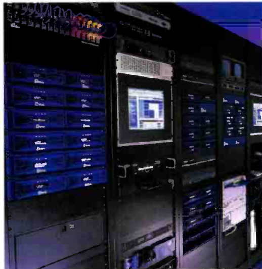
Minerva's IPTV encoders and decoders are being used by Hargray, a local phone company in the Hilton Head Island area of South Carolina.
