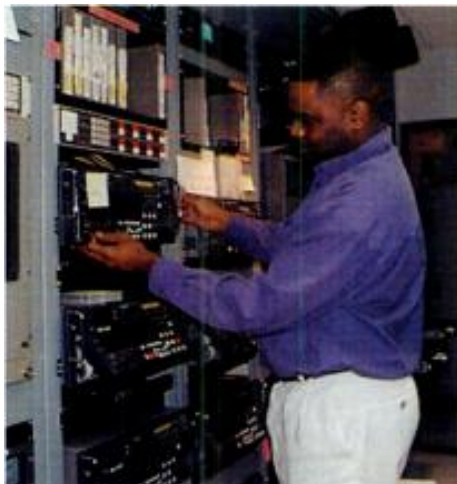
Corey Tutt, a C-SPAN engineer, installs one of the network's new Panasonic DVCPRO decks.
