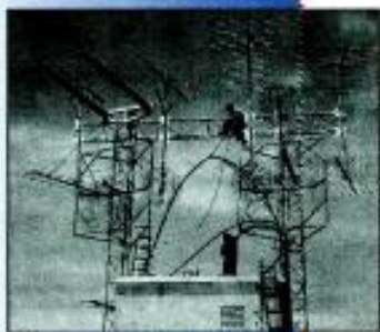
Microwave antenna tower
