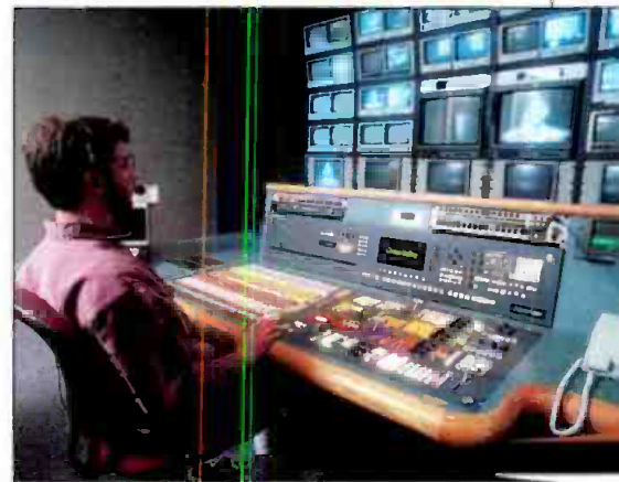
A Grass Valley 4000-3 digital switcher directs traffic in production control.
