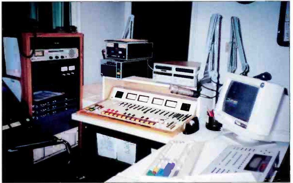
The remodeled production studio for WYRK(FM) Buffalo with new computer systems and broadcast console.
