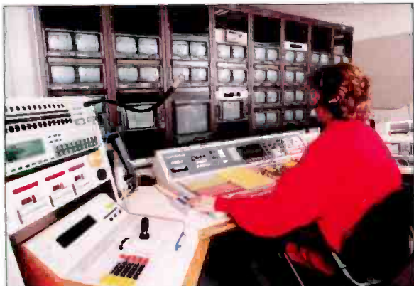
The all-digital production control room is built around a Grass Valley 400-2 switcher and Neve audio console.
