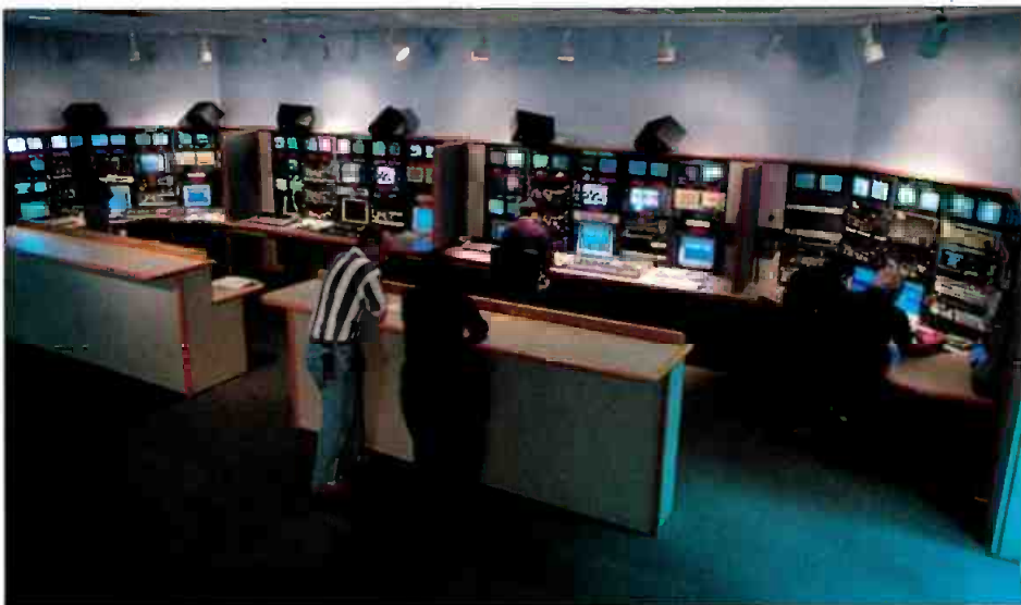
The facility's master control center (right) has four separate operator stations.
