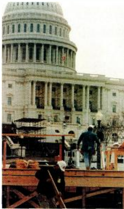
Workmen were up early every morning last week to construct camera stands and other structures for TV coverage of the Clinton-Gore inaugural on Jan. 20.
