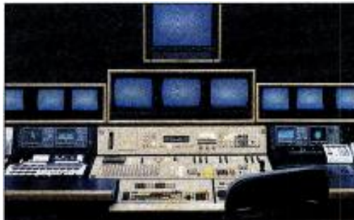
DIGITAL FINISHING ROOM
