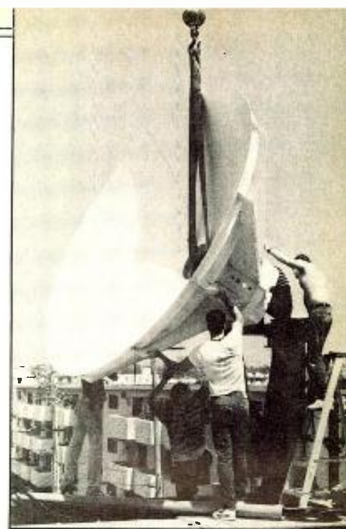
IDB erects earth station at Los Angeles International Teleport to bring in feeds from the Olympics
