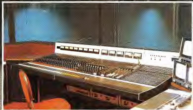
WBS 800886 Audio Console overlooks Convention facilities.
