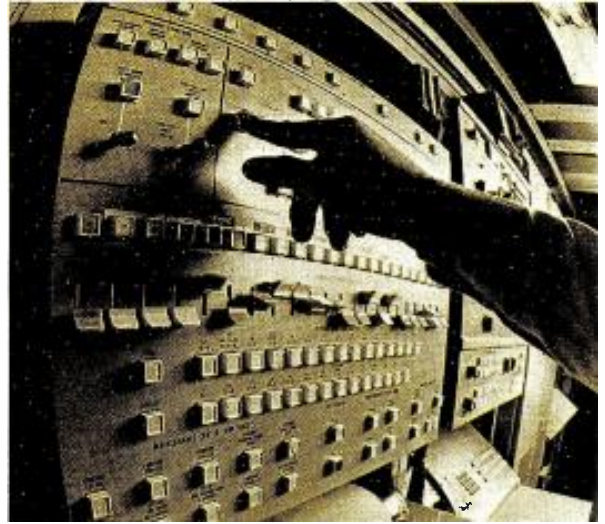
Electronic switching systems, a thousand times faster than the equipment they replace, are now being installed across the nation.
