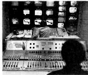
ONE OF FOUR SEPARATE CONTROL CENTERS.
