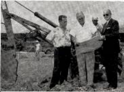
AT the excavation site of the new $150,000 plant KONA (TV) Honolulu is building, executives stop to review plans. They are (l to r) Lorrin P. Thurston, chairman of the board, and John D. Keating, president-general manager of the station. December is target date for KONA's new facilities.
