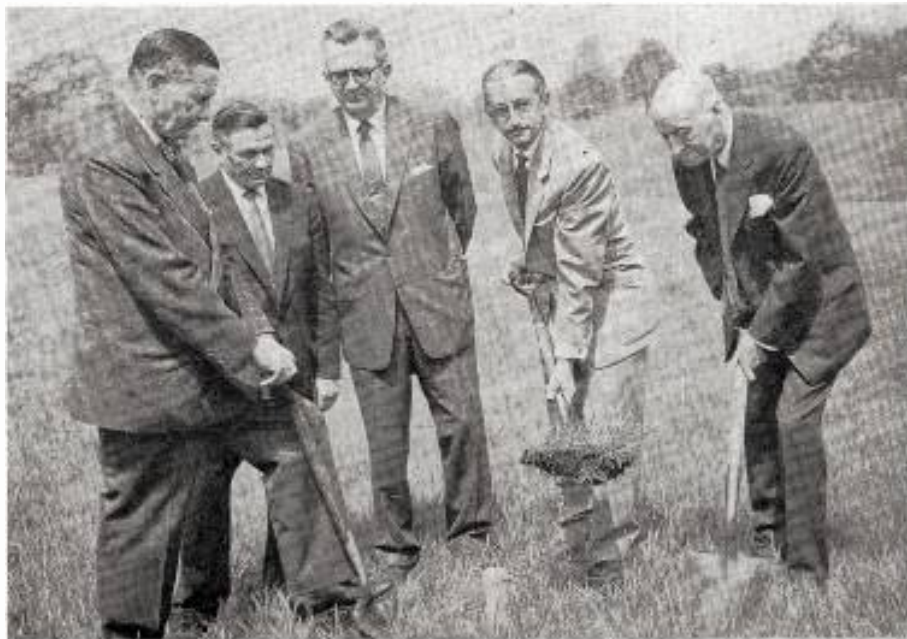
SOD-BUSTERS break ground for WHDH-TV Boston's new tower. L. to r.: Robert B. Choate, WHDH president; Philip K. Baldwin, chief engineer; Jack O'Brien, RCA northeastern regional manager; William B. McGrath, WHDH vice president, and Sidney W. Winslow Jr., president of the Herald-Traveler Corp. Boston's fourth vhf outlet is expected to be on the air on ch. 5 before Christmas.
