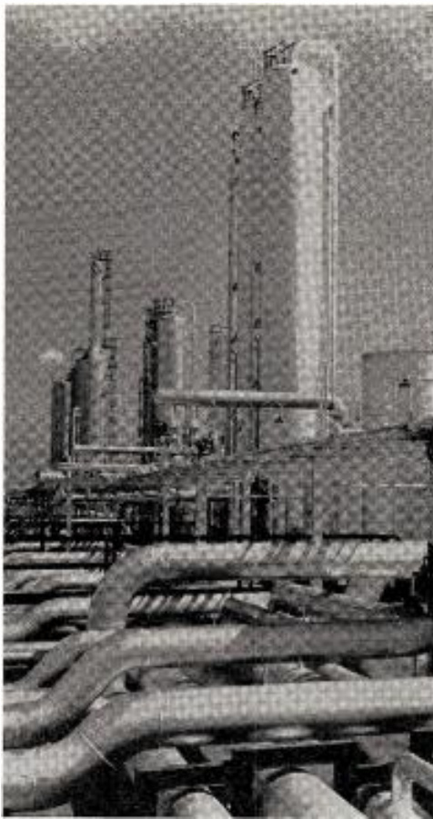
TWENTY PERCENT of the nation's crude oil is produced south and west of Lubbock, with reserves estimated at billions of barrels. This is the Stanolind plant.
