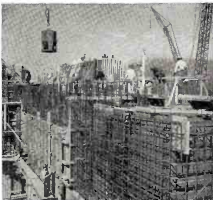
First Atomic Power Plant is being built near Shippingport, Pa. This tremendous project uses thousands of tons of concrete—all reinforced with steel bars and mesh from U.S. Steel Supply.
