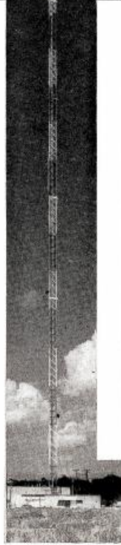
Typical Emsco guyed TV tower, Houston, Texas
