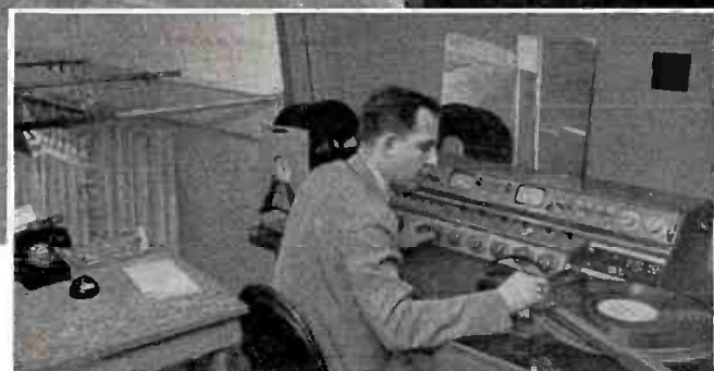
Chief Engineer Miller checks audio levels on Altec 250A speech input console. Distributed by Graybar, this completely self-contained unit provides all necessary monitoring, cue, audition, and signaling circuits for WNAO's audio control.
