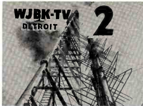
HERE is an ID shown on WJBK of its new tower while it was under construction. The station has recently concentrated on promoting the 1,057-ft. structure.
