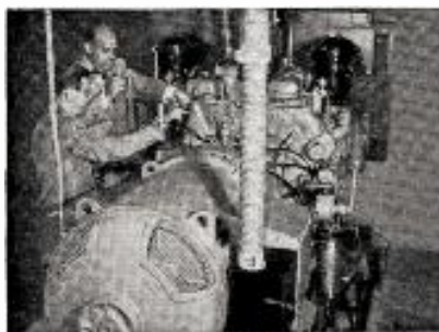
WJR—Detroit, Michigan, uses 200 kw. GM Diesel generator set as stand-by power for 50,000-watt transmitter. Compactness of unit permitted installation in garage adjoining transmitter building—eliminating cost of a specially designed building.
