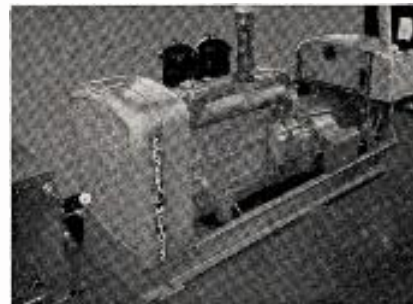
WKTV—UTICA, N. Y., uses a 100 kw. General Motors Diesel generator set for stand-by power. Set can be started remotely from the control room. Low vibration characteristic of engine permitted installation in room adjacent to transmitter and within 30 feet of studio.
