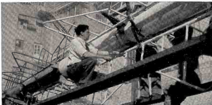
Clem Castle, Storer Broadcast Company engineer, inspects the General Electric 6-Bay Antenna before hoisting to the tower.
