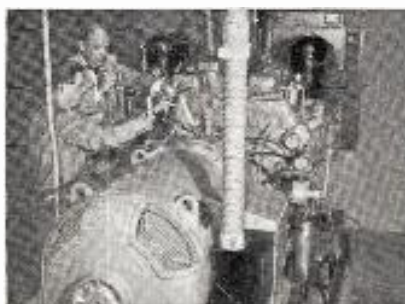
WJR—Detroit, Michigan, uses 200 kw. GM Diesel generator set as stand-by power for 50,000-watt transmitter. Compactness of unit permitted installation in garage adjoining transmitter building—eliminating cost of a specially designed building.
