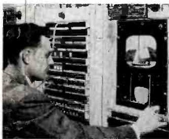
AT OPERATING control position at new TV network center in New York, a technician tests, maintains and switches network channels interconnecting local television studios with Bell System's inter-city hookups. Fidelity of both video and sound transmission is checked with built-in picture tubes, oscilloscopes and loudspeakers at each monitoring position.
