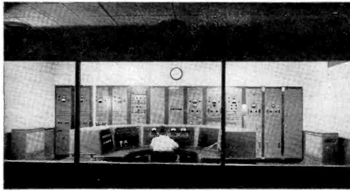
RADIOCENTRO master control which feeds CMQ, along with seven stations on its network (which have no local studios) as well as three stations under Mestre ownership in Havana. A fourth channel is available for another Havana station.
