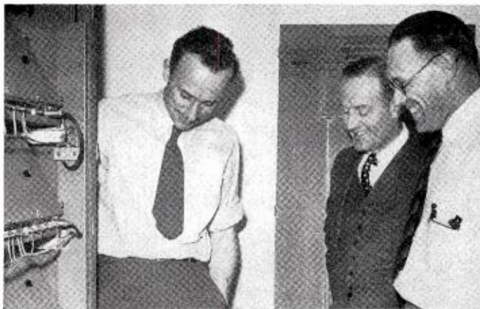
SMILING APPROVAL of the new 50-kw. transmitter for W45D, FM station of the Detroit Evening News , is given by Frank Gunther, vice-president of Radio Engineering Labs., Long Island City, N. Y., who supervised the installation of the transmitter; William J. Scripps, general manager of WWJ, the News standard broadcasting station, and Carl Weiser, chief engineer of W45D.
