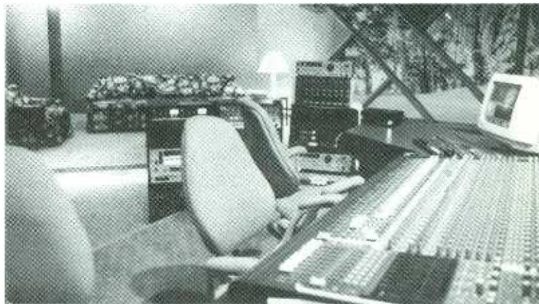
Studio Morin Heights' Far Side is a veritable control room with a view, offering producers and engineers a hi-tech environment in a natural setting.
