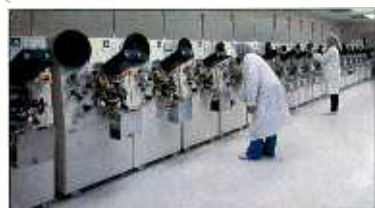
Master Control ■ High resolution monitors and top of the line source VTRs are constantly monitored for optimum performance.
