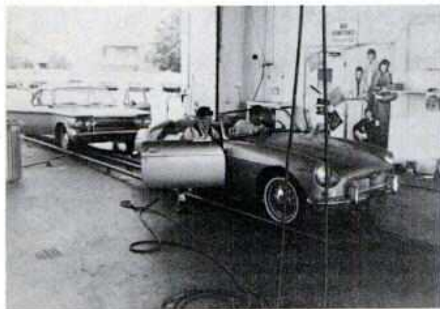
CONVEYOR BELT SYSTEM is used by Muntz Stereo Pak to attain maximum installation efficiency for tape CARtridge installations. The location is being set for a capacity of 150-175 player installations per day.
