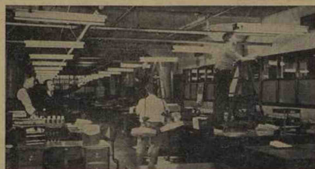
"THE EYES HAVE IT" at the general offices of the Rock-Ola Mfg. Corp., where an elaborate new lighting system has been installed. "Our primary purpose in installing this new fluorescent lighting system is to improve working conditions for Rock-Ola employees whenever and wherever possible," declared H. Ber, Rock-Ola controller.
