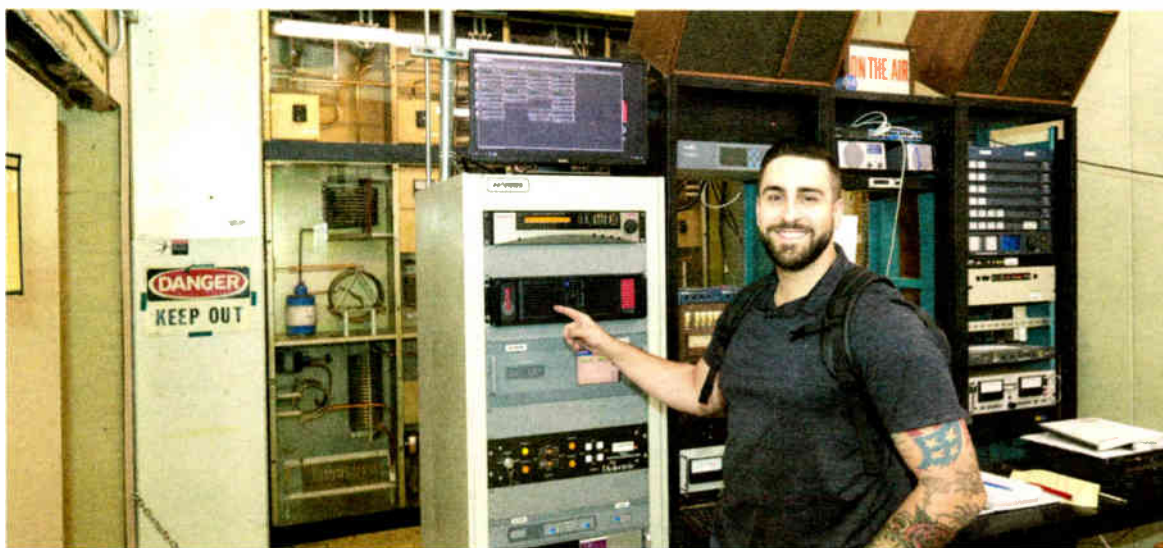
Jason Ornellas, Bonneville's regional director of engineering for the West Region, is shown at KHTK(AM) Sacramento with the XPN-AM processor.
