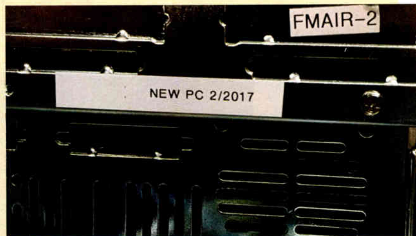
Fig. 3: Label computer hardware to keep track of aging equipment.
