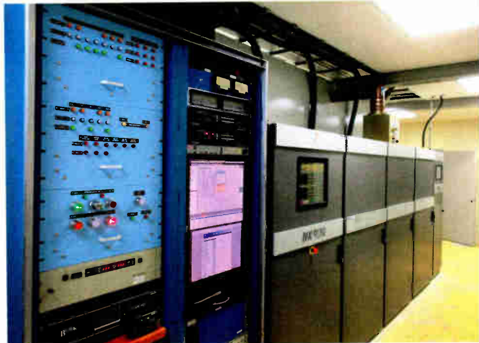
The new transmitter and associated equipment.
