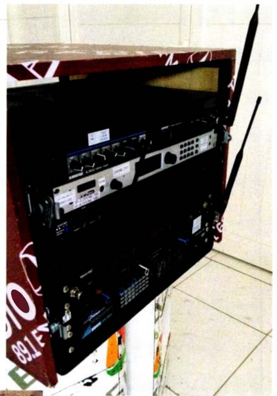
The equipment rack with the Telos Z/IP One in the center.
