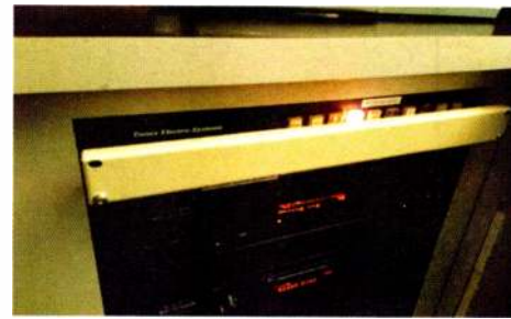
Fig. 3: A blank panel mounted on long standoffs prevents switches or other front-panel components from being bumped by the studio chair.
