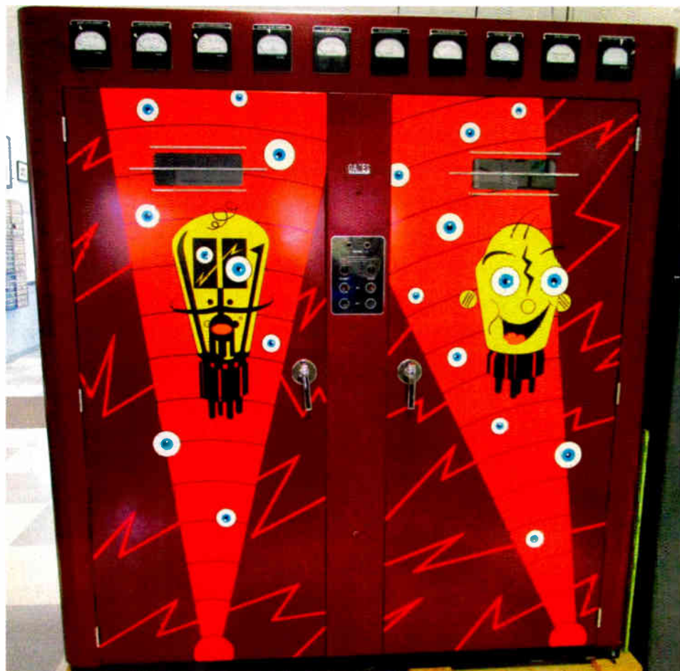
Not all of Moersdorf's transmitters are kept "stock," as exemplified by this now one-of-a-kind Gates BC-1F 1 kW model from the early 1950s. (Moersdorf has another with Parker Gates' factory paint job.)
