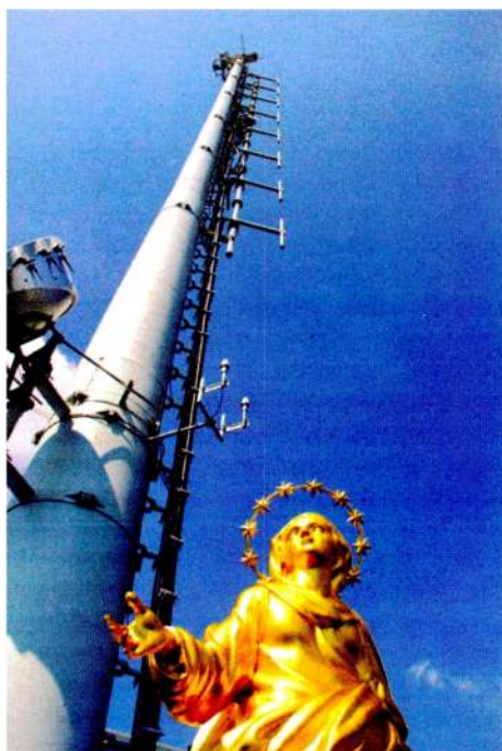
The high-power FM antenna Aldena recently installed for network operator Raiway in Milan.
