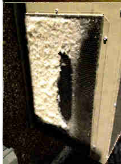
Fig. 3: The screen is nearly completely clogged.
