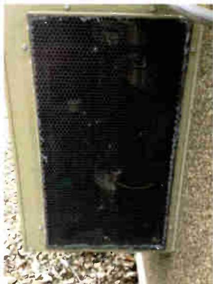
Fig. 1: A fiberglass screen keeps cottonwood seeds out of the air conditioner.
