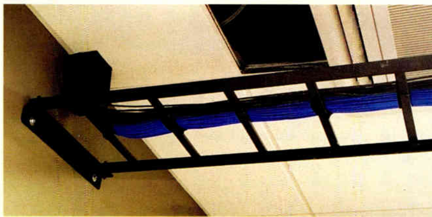
Fig. 3: A square conduit at left channels Cat-6 cable into the plenum ceiling.
