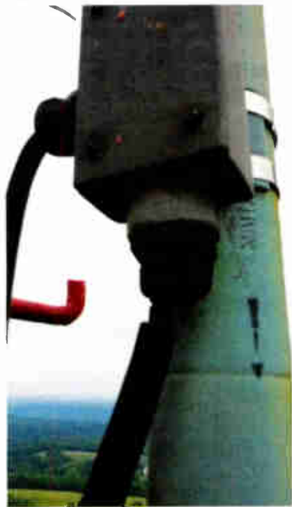
Fig. 3: Aquaseal and multi-use electrical tape can provide a temporary repair for an antenna heater cable.
