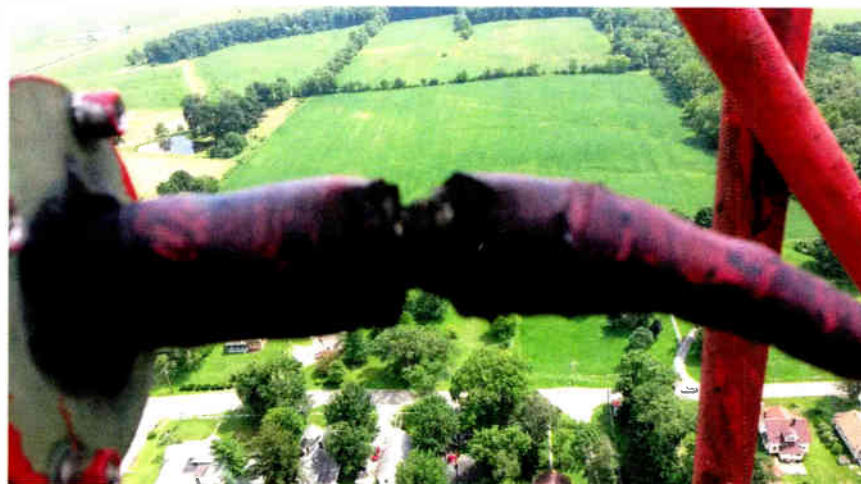
Fig. 1: A cracked antenna harness is visible in the foreground of this image taken during a re-lamp visit.
