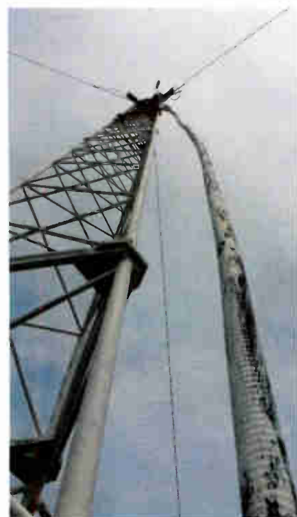
Fig. 4: Unsecured coax blowing in the wind eventually will fail.
