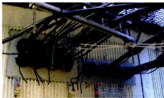
Fig. 3: Tinned copper bus bars are avoided by copper thieves because scrap facilities don't want them.
