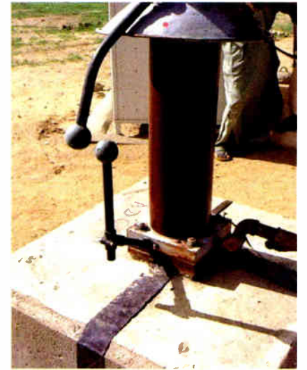
Fig. 2: Check the tower base spark gap, making sure the balls are smooth.
