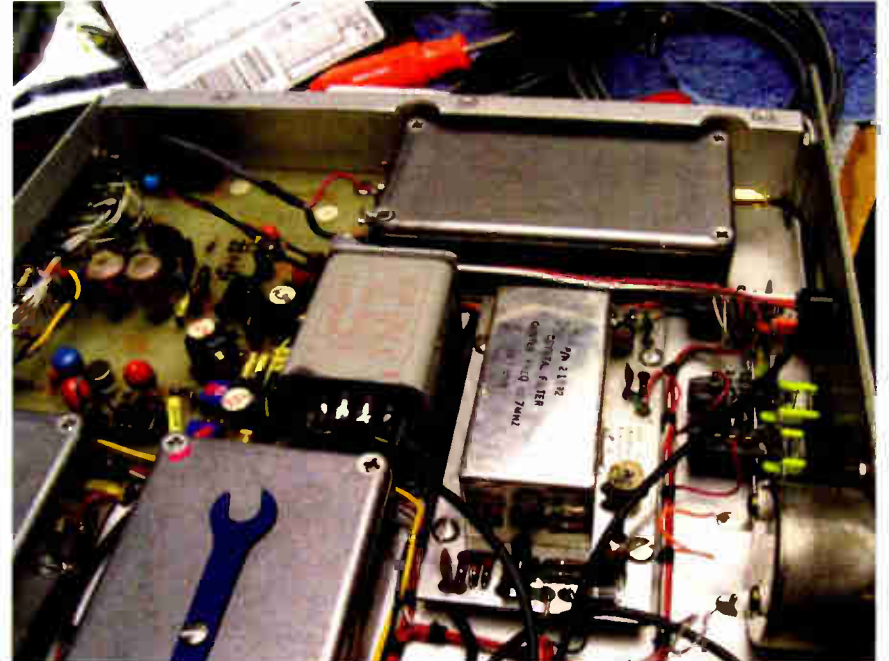
Fig. 2: Inside the Moseley RPU, showing the overall modifications
