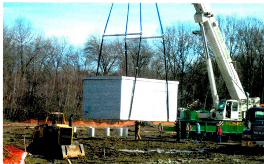
Pre-cast tuning houses were 14 by 20 feet and each weighed 60,000 pounds. To keep them up out of the flood plain they were set on caissons that were 3 feet in diameter below grade and 1-1/2 feet diameter above grade. Temporary roadways were built to support the crane and trucks carrying the buildings; the roadways had to be removed after construction to restore the wetlands.
