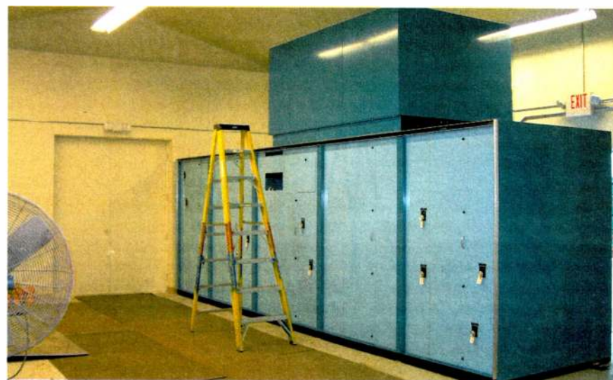
Photos from the Boston area triplex project. This is the WKOX phasor. 'The building footprint couldn't be enlarged,' Warner said, 'so I specified cantilever trusses to create a cathedral ceiling so we could make the phasor two stories high.'
