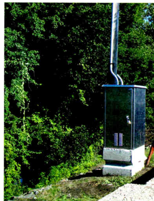
Fig. 3: Same station, after the upgrade ...
