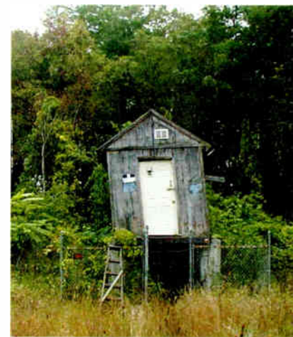
Fig. 2: Some towers are hazardous to climb. This building looks hazardous even to enter.
