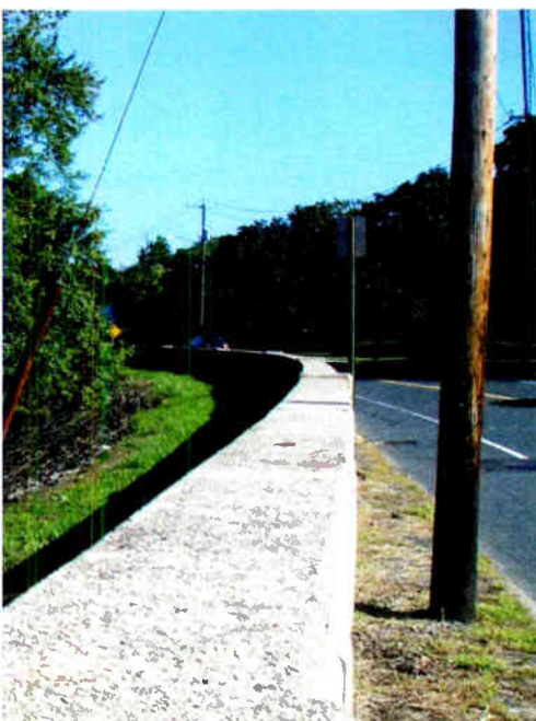
No termites eating this enclosure!
