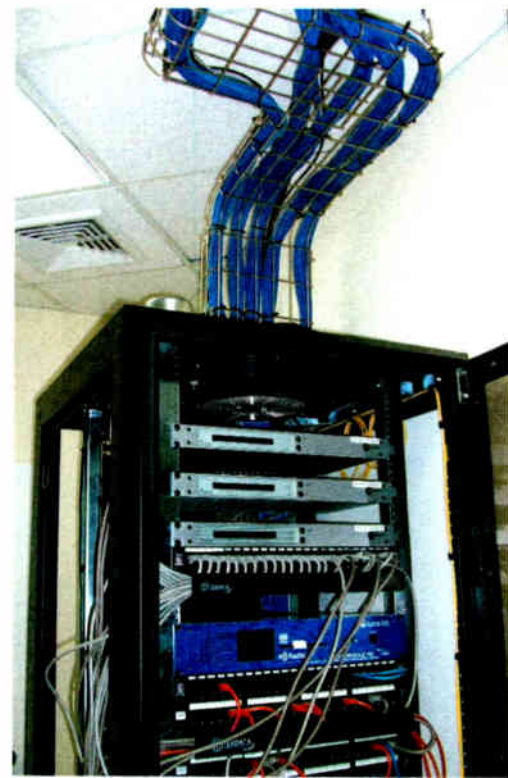
Master Control Rack with Cat-6 cables entering from the studios.
