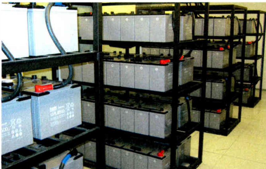
UPS on steroids: RFE/RL's basement holds enough backup charge and emergency cooling to keep the most important systems operational during even lengthy outages.
