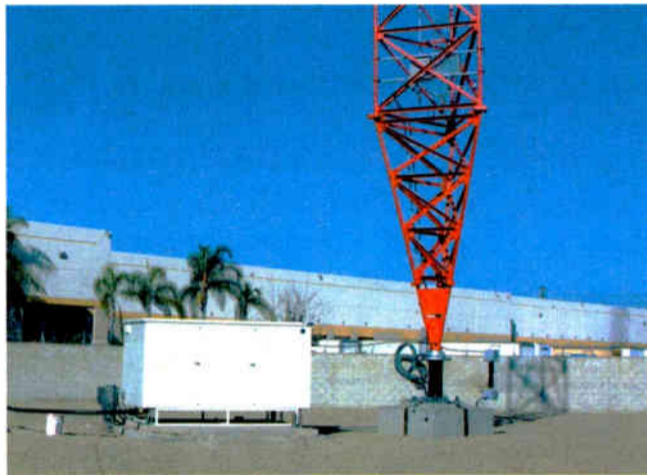
New antenna tuning unit and base insulator of the replacement KFI tower.
