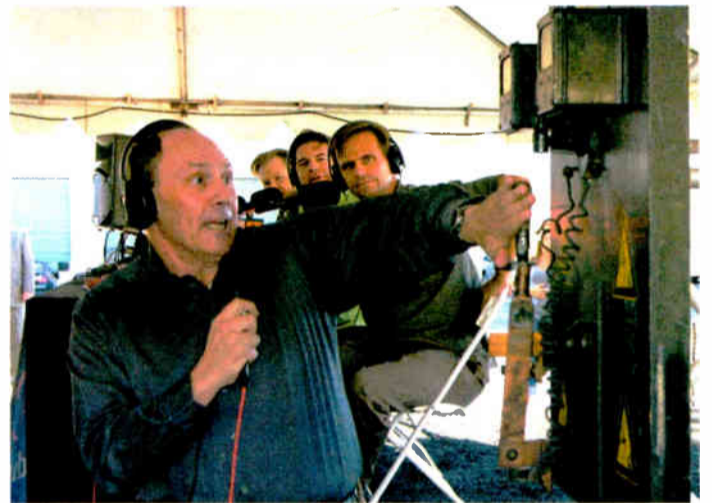
Morning host Bill Handel, closing the ceremonial knife switch, puts KFI on full 50 kW power into the replacement tower.
