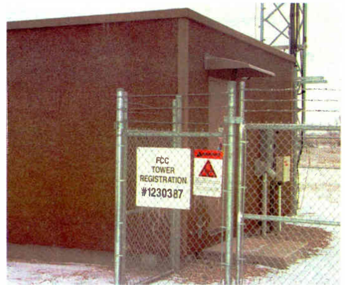
Fig. 4: A properly identified tower. Note both the ID number and Rad-haz sign.
