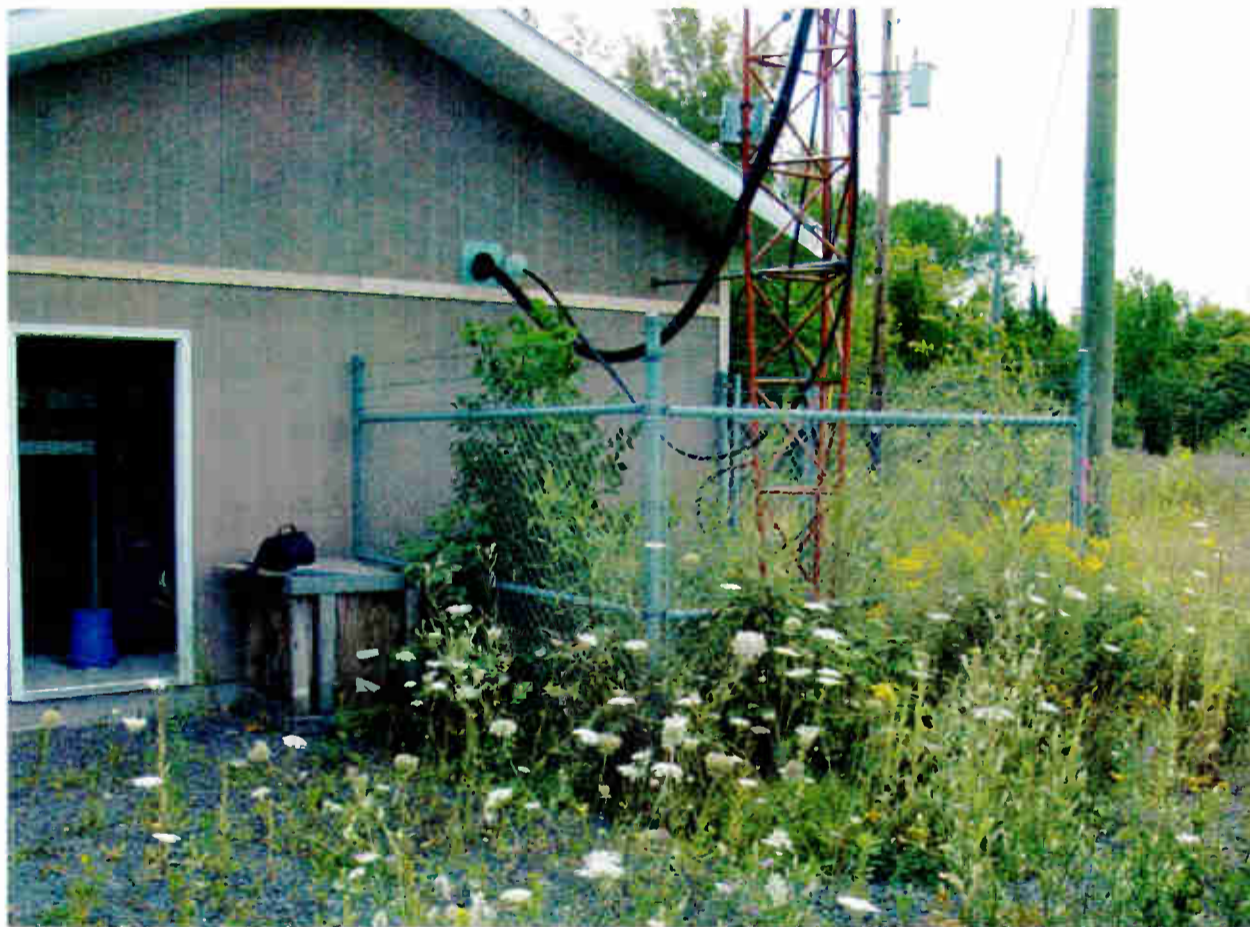
Fig. 1: How many problems can you spot in this photo?
