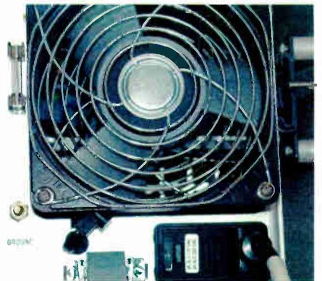
Fig. 2: Keep fans and filters clean, like this exciter.
