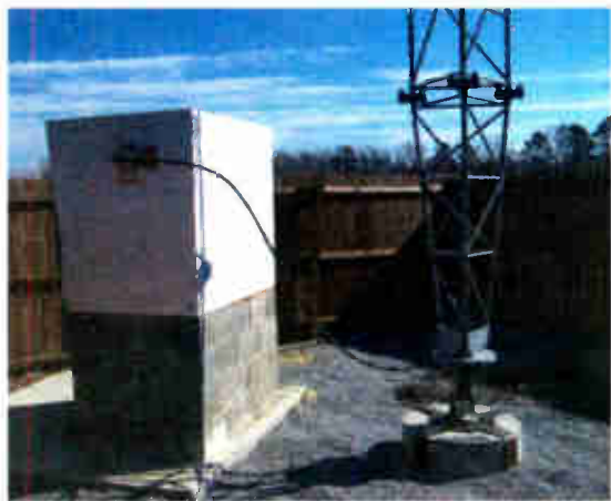
High-Power Antenna Tuning Units
