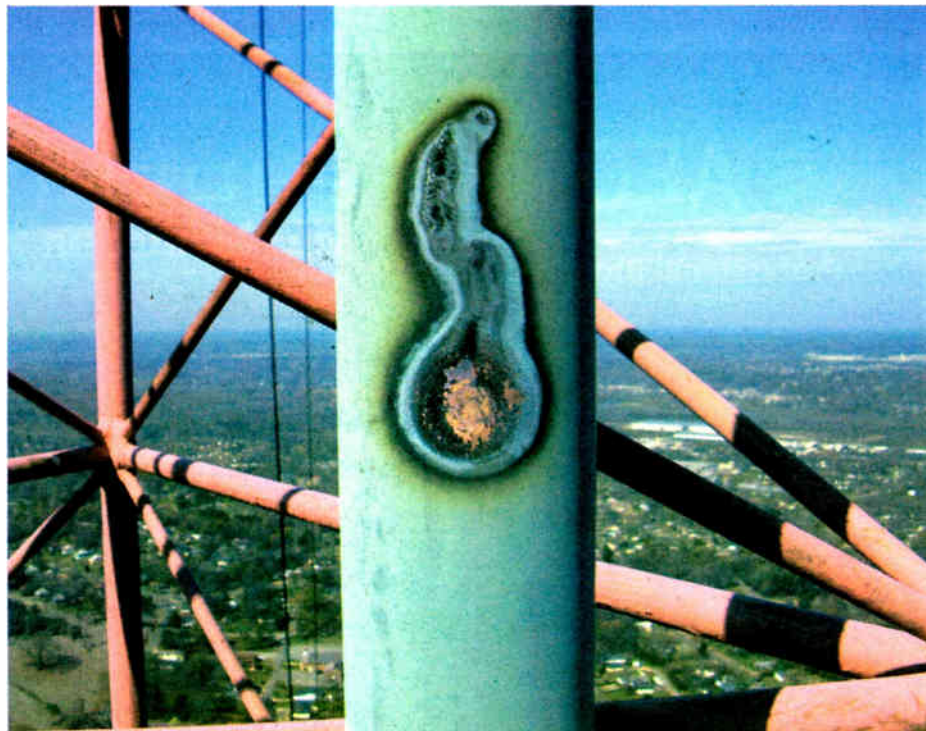
A direct hit to the antenna produced 'collateral damage' down the transmission line.
