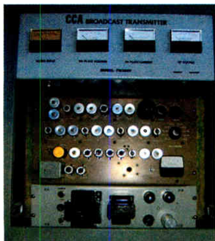
This CCA FM-10DT served as the original WDCV(FM) transmitter and is now a backup. It is fully operational.
