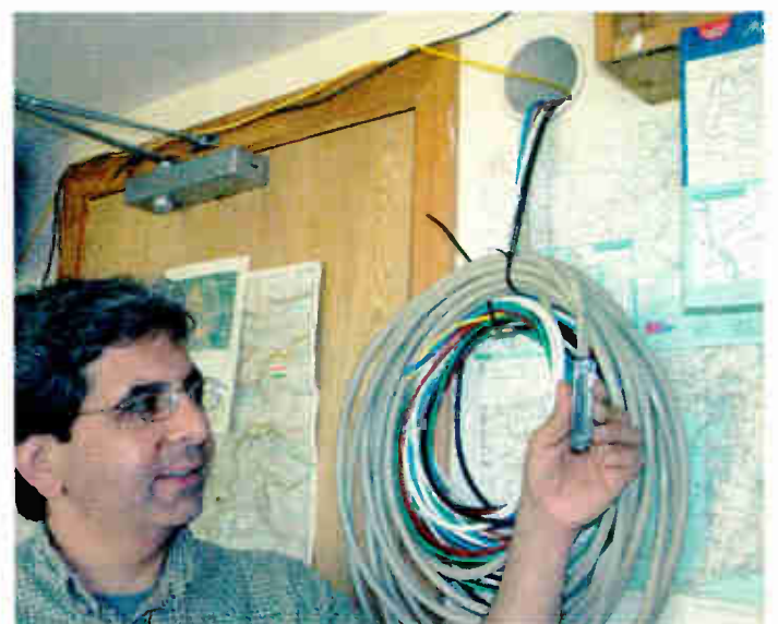
Fig. 3: The raceway entry into the studio has room for plenty of cables.
