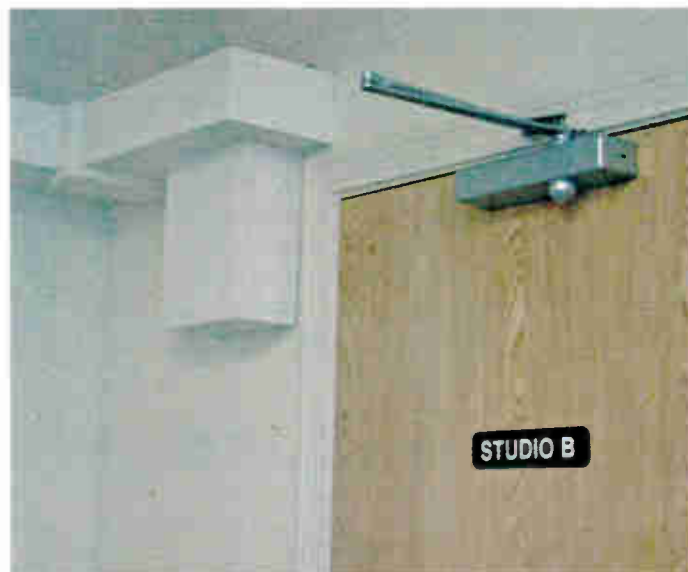
Fig. 2: At the studio entry, a box drops the cables down and through the wall.
