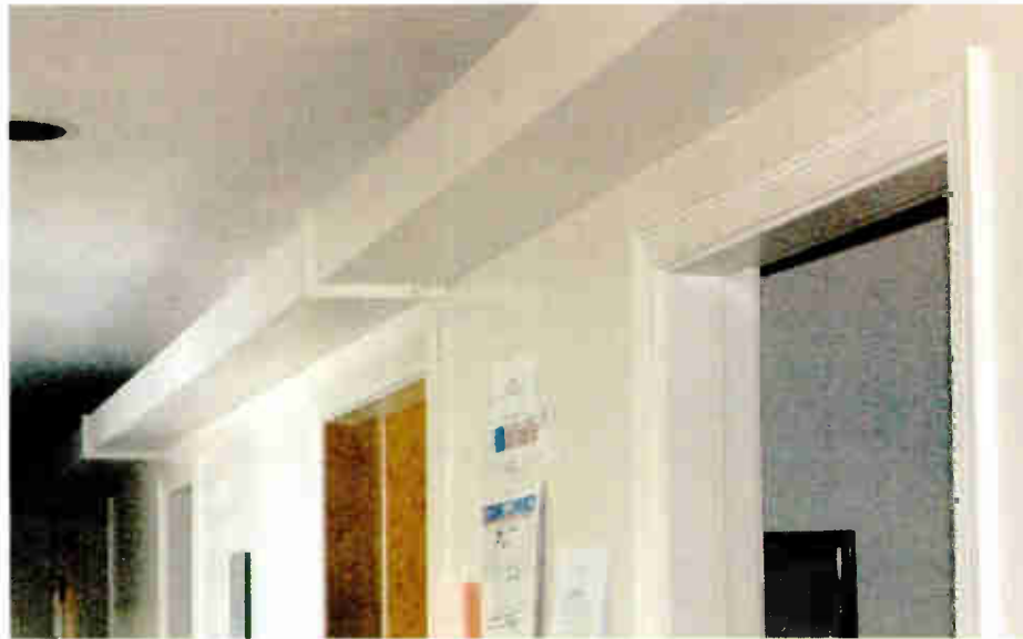
Fig. 1: A wooden raceway runs the length of the hall and holds interstudio cabling.
