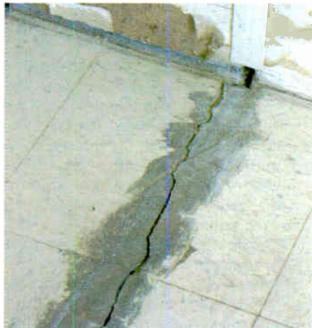
Fig. 6: Don't disregard settling cracks that may get bigger and pose a leak threat.
